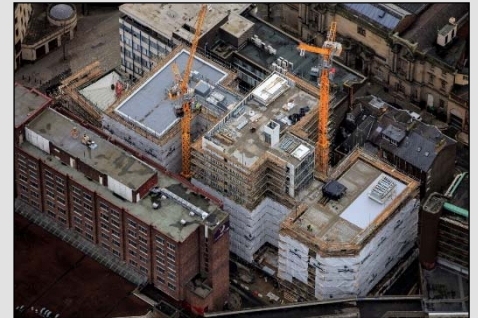
Aerial view of the ongoing installation in the heart of the city centre
