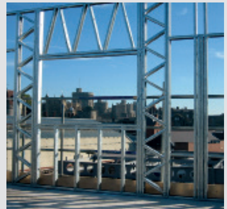
Light steel load-bearing wall with lintel formed from a light steel truss
