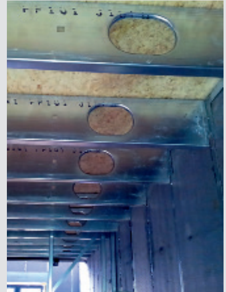
Large holes in light steel floor joists for integration of services
