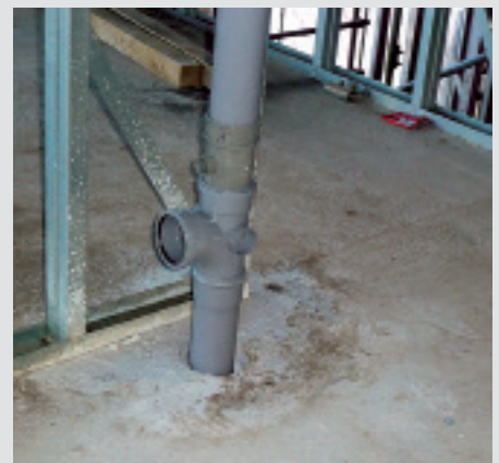
Individual opening for service pipe formed in a composite slab (maximum 150 mm diameter)
