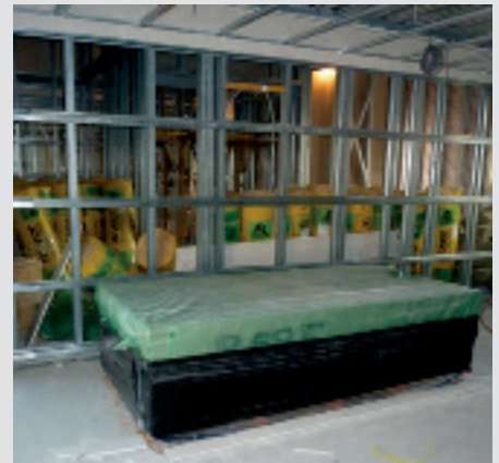
Construction materials stored on the floor of a light steel frame building
