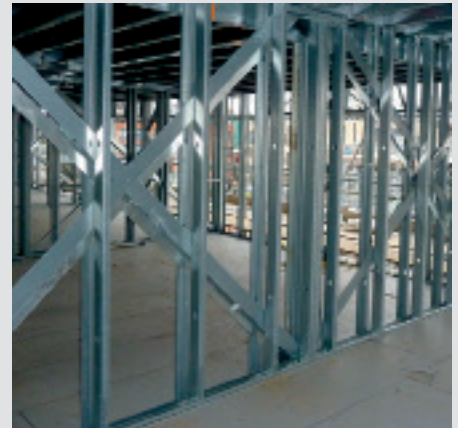
Cross-bracing in light steel frame walls forms a vital part of the frame stability
